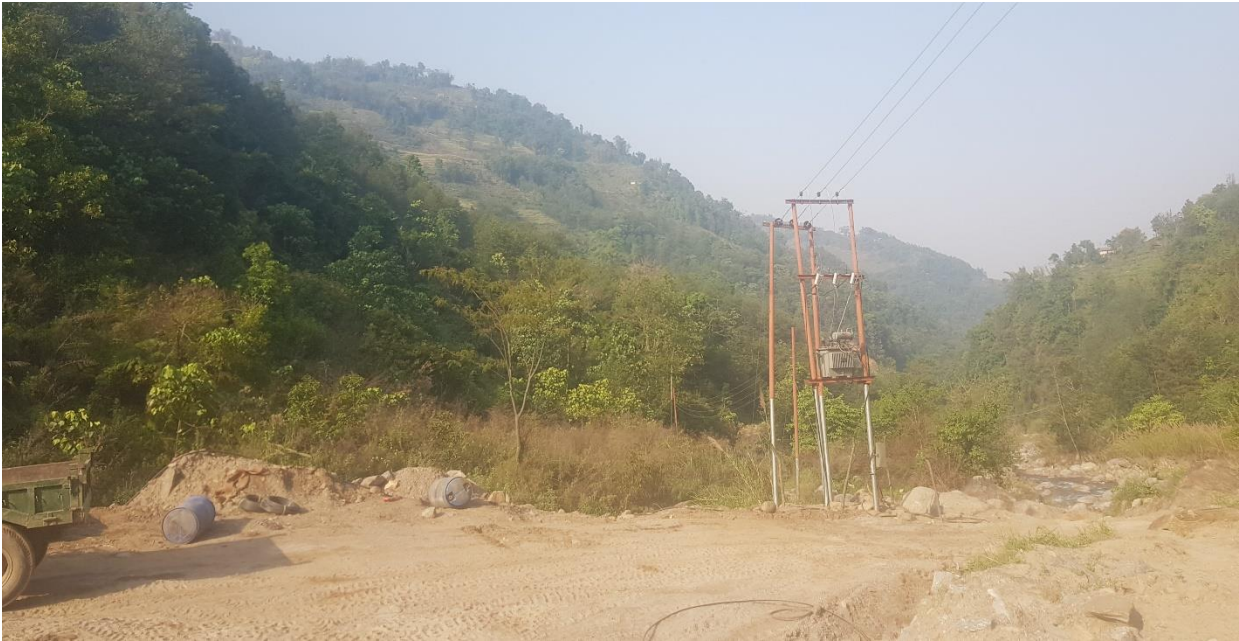
Figure 13: Transformer for construction power
